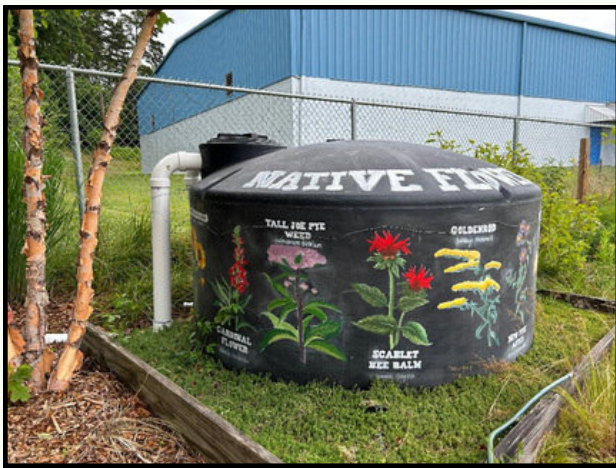
A roof-harvested rain collection system
